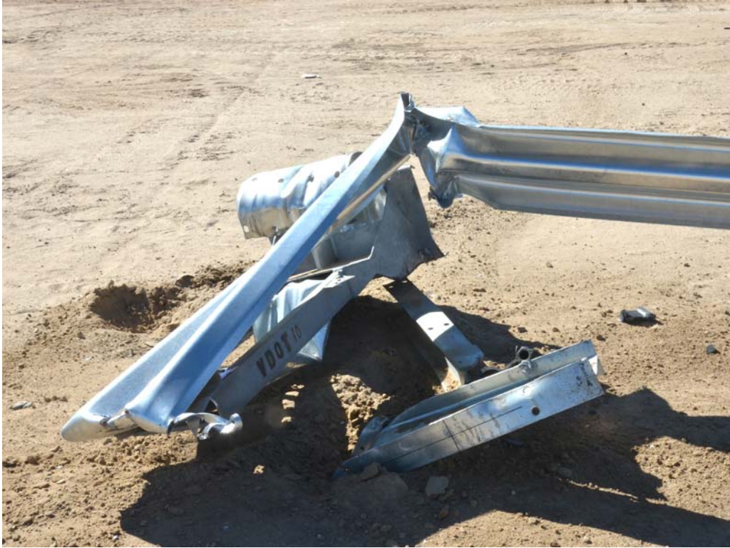
FIGURE 35. Test Article Damage
