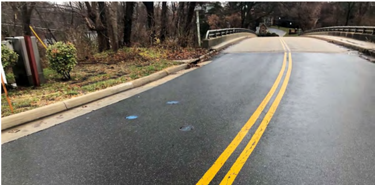
Figure 11 – Underground Utilities and Gas Monitoring Station on South-West Corner of the Bridge
